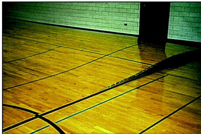
Figure 6: Maple flooring after high humidity.
