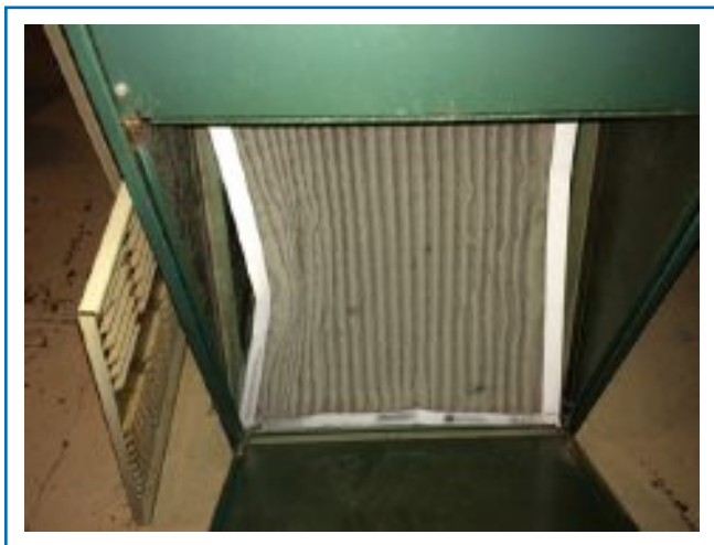
Figure 8. Example of large amounts of bypass airflow around a filter in an air-handling unit because of improper installation combined with excessive loading that increased the pressure drop across the filter beyond what the filter was capable of supporting. Photo credit: Brent Stephens.
